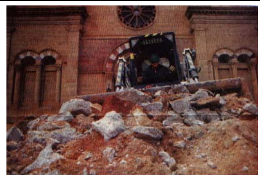
Demolition in front of St. Francis Cathedral, Santa Fe as part of remodeling work that will include construction of a labyrinth.
